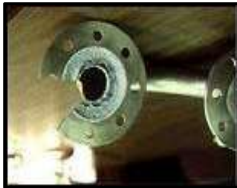
Fig. 5 Concentration cell corrosion
